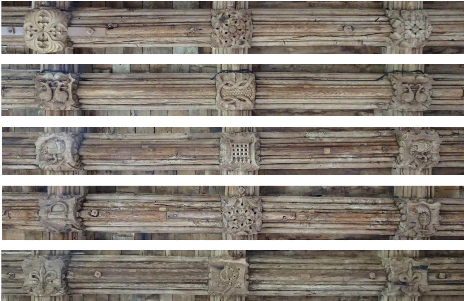
Roof bosses in the south aisle of Thaxted Church. From the top (east): double rose flanked by foliage; Bourchier knot flanked by water bouquets; portcullis flanked by pomegranates; double rose flanked by fetterlock and ostrich feather; pomegranate impaling rose flanked by fleur de lis. Other bosses further west not illustrated.
