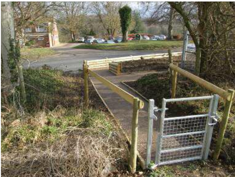
The new gate, with the Golf Club across the road in the distance
