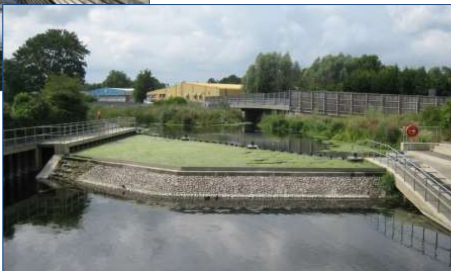
Left: Chapel Arches basin, and below: Boat Lift and Weir, on 27 th July, with a mat of blanket weed between the boom and the weir
